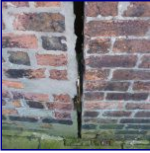
Rod Cox's Brick wall, near Rufus Court. The crack between the brick wall and the gabled building.
