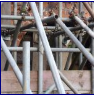
Rod Cox's Brick wall, near Rufus Court. Picture taken from Abbey Green. The scaffolding supporting the collapsing brick wall.
